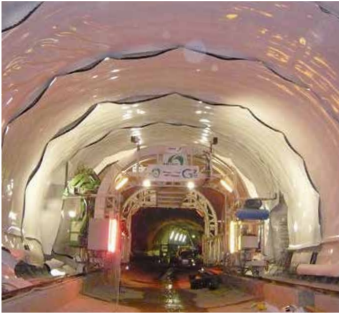
Tunnel, PVC 0.1 inch (2.5 mm)
